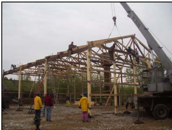
Erection of a "pole barn" structure at the rehab work center in Turbov.
